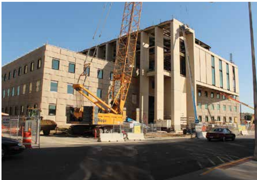
Two color variations were created for the precast concrete panels by changing the sand ratio in the mix. That change created a golden “Yellowstone” color as well as an offsetting “traditional government white.”
