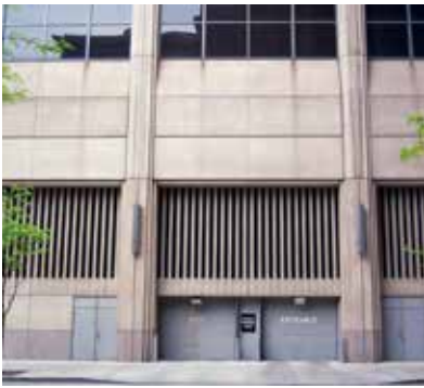
Figure 4 (b) Water flow over glass depositing dirt soiling pattern.
