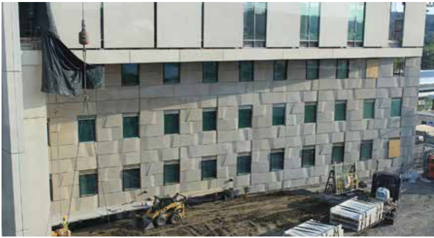
In some areas on the first level, recessed façades required the precast concrete panels to be set first so steel could be erected over them. Close cooperation on such issues allowed the project to be completed in a record-setting 27 months.
