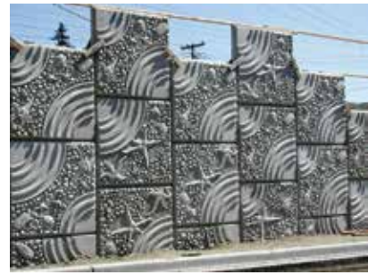
Puzzle-piecing is a technique in which one form is used to cast a number of panels, but the design is turned 90 or 180 degrees to create a less repetitious pattern. This design was used on a highway ramp in Shoreline, Wash., with designs by Vicki Scuri of Siteworks. Photo: Scott System.
